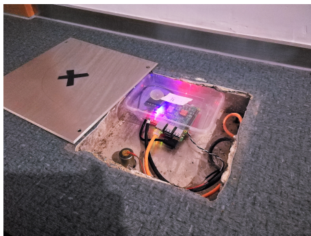
Figure 3: Deployed sensing unit example: For safety reason, sensing unit is installed underneath the floor, and covered with a steel plate. The geophone sensor is fixed on the floor to ensure a stable connection.
